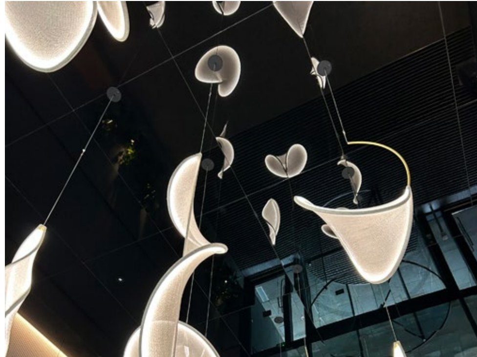
Decorative, feature lighting to double height space at ground level
