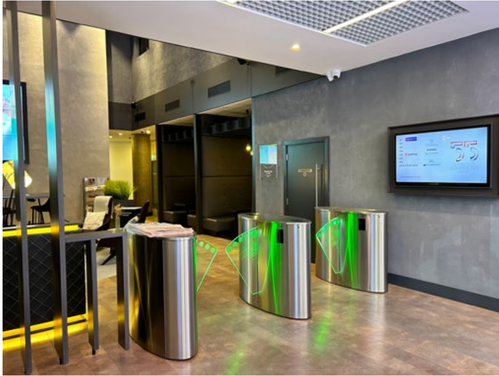
Ground floor speedgates next to reception
